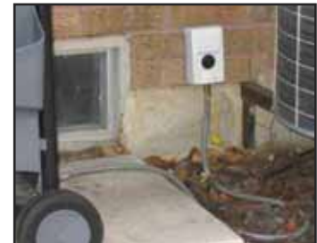
Hose Assembly Length Restrictions May Apply: Check with Local Jurisdictions
