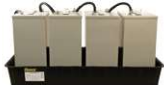
Battery tray with four L16/GC2 batteries 120220
